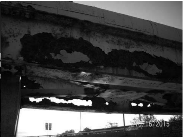
Close-up of holes in web, looking east
