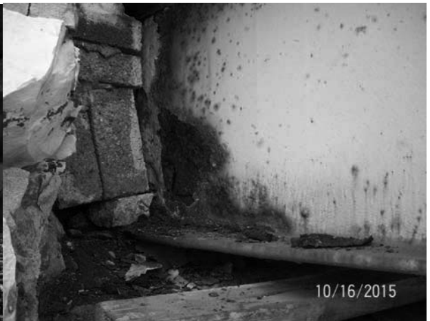
Hole in right girder web at South Abutment
